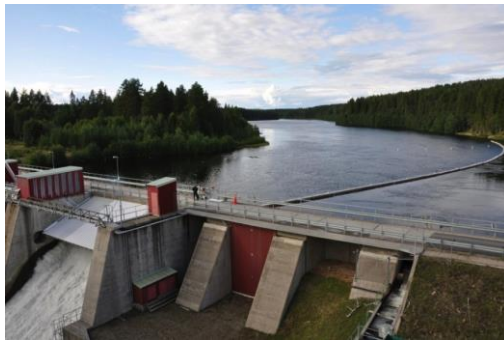
Fig. 1. View of part of a dam, a spillway (bottom left) and a smolt guiding device that stretches over the water. Most water goes to the turbines that are located underground and to the right of the picture.
