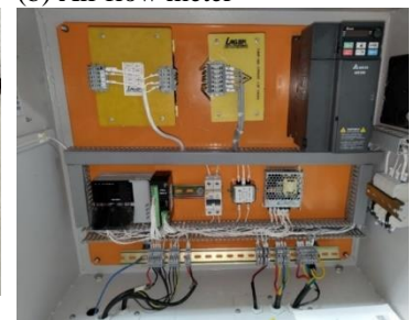
(e) Control panel with VFD
